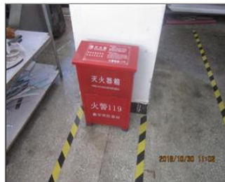
Photo of fire safety equipment Fire extinguishers.JPG
