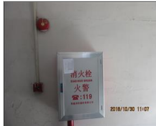
Photo of fire safety equipment Fire alarm and fire hydrant.JPG
